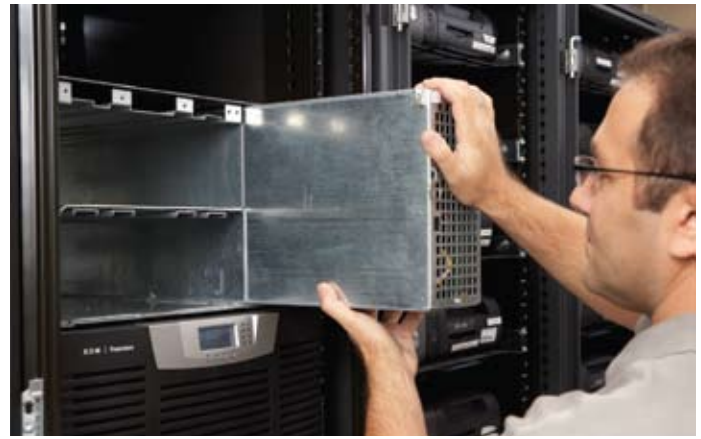
IT staff can easily install electronics modules.
