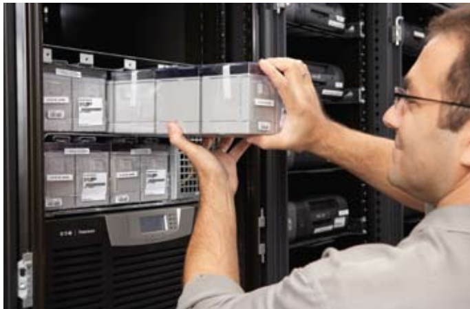
IT staff can easily replace battery modules.
