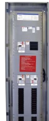
Wall-mount maintenance bypass panel
